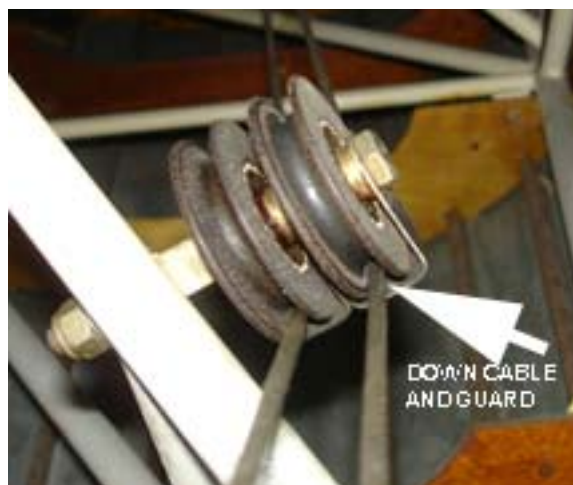
Fig. 1 Elevator Cable Pulleys at Station 212
